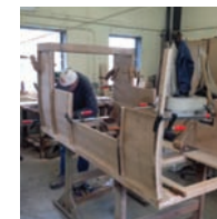
Dick Anderson clamps a side board to a vertical riser mortised into the floor sill.
